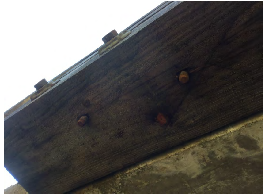
Guardrail missing some hardware
