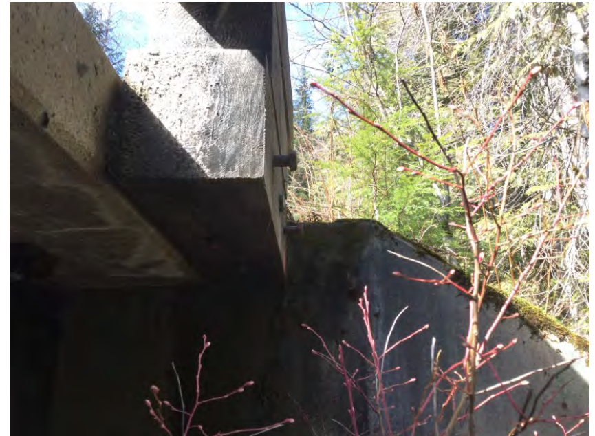
Loose sideblock bolts
