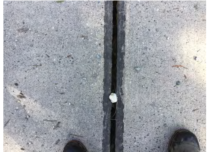
Deck joint seals missing
